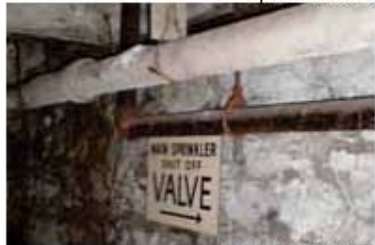
c) basement sprinklers
